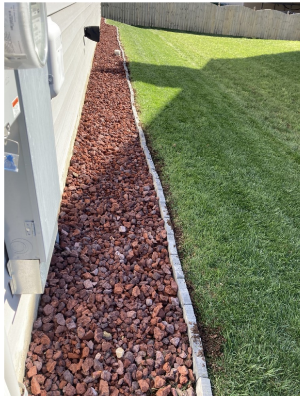
Figure 4. Placing rock or other inorganic mulch next to the foundation base should reduce the risk of clover mites wandering indoors. Credit: email submission.
