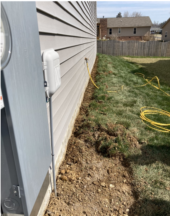
Figure 3. Lush grass being removed 2 ft. from the foundation. Credit: email submission.
