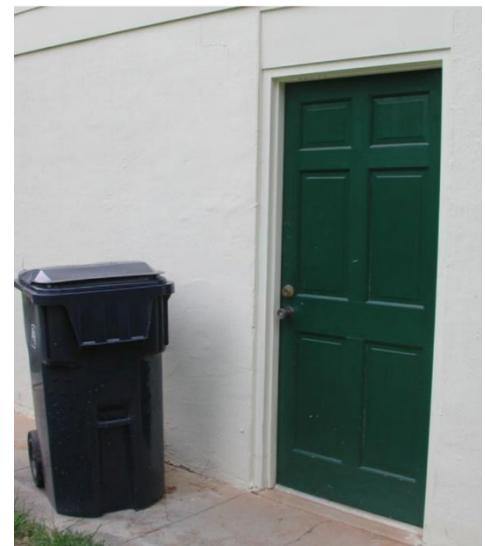
Figure 8. Move garbage cans away from the structure. Ants overwintered in the door frame and moved under the garbage can when temperatures warmed in the spring. Photo: UT E&PP
